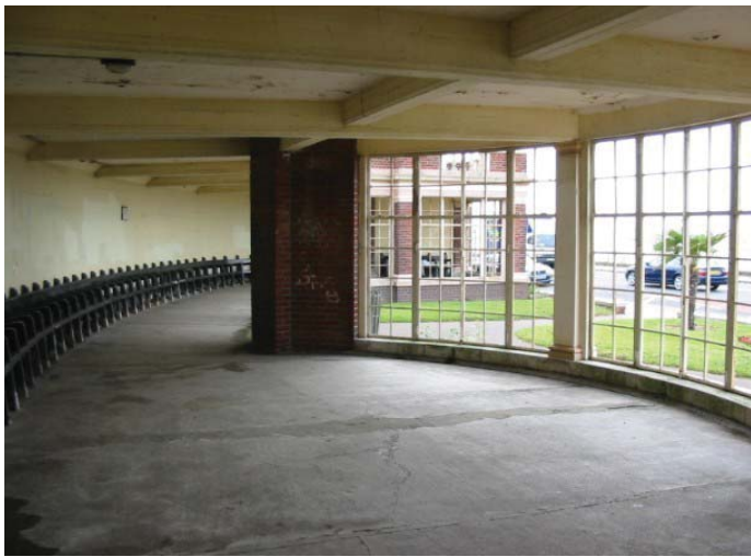
View inside shelter
